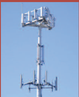
Telecommunication devices, aerials and phone masts.
