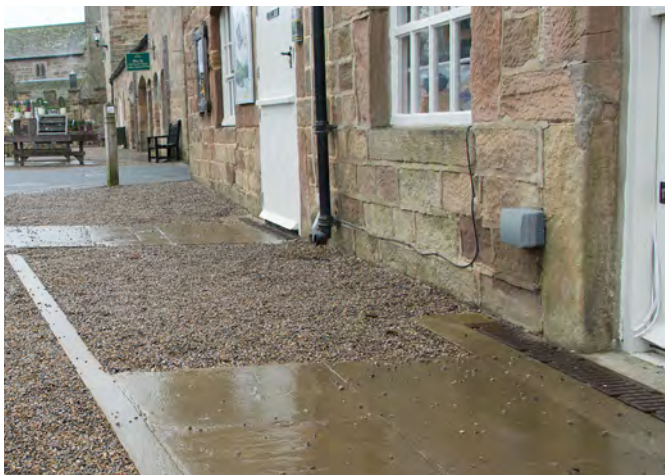
A mixture of surfaces can be challenging, and gravel can migrate making other surfaces more hazardous.
