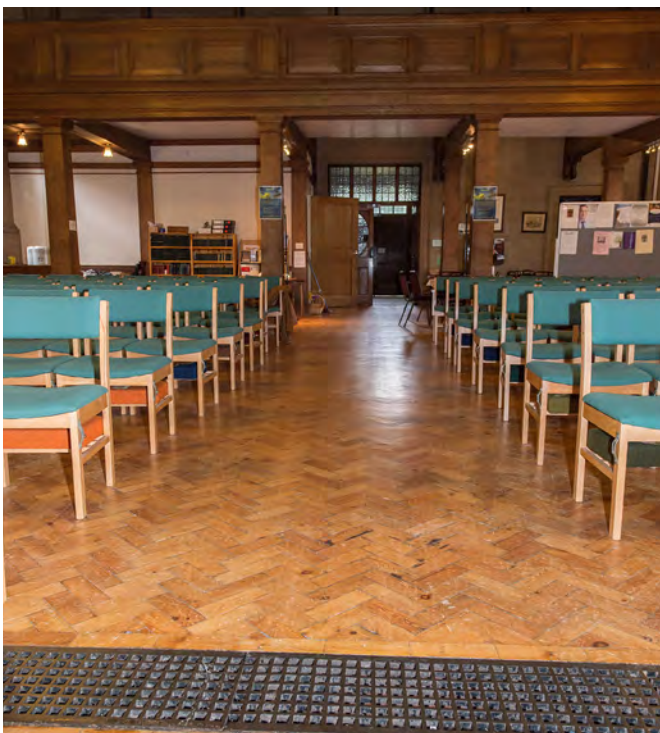
Different types of flooring that are adjacent to each other may pose a slip hazard if they present unexpected changes in slip resistance.
